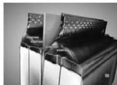
Battery inspection for Overhang Distances
